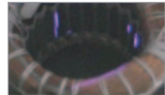
Figure 8: Corona discharge in motor
